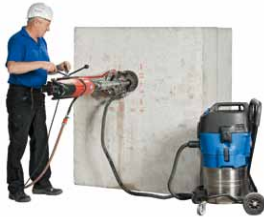
Red markings indicate the position of the reinforcement. Avoiding damage to the reinforcement through drilling the core hole between the reinforcing rods.
