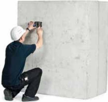
Using a reinforcement scanner to determine the existing reinforcement in the construction component.
